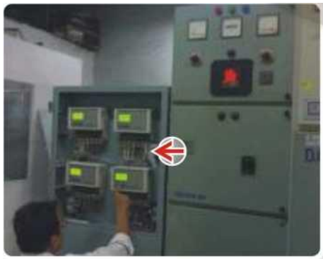
Genset Efficiency Monitoring HLL Urai, M.P.
