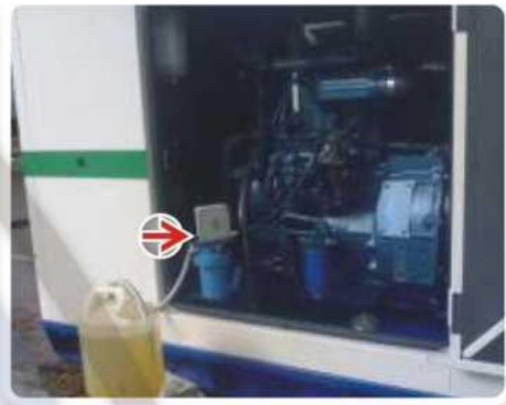
15 KVA Genset Fuel Monitor Accuracy Validation KOEL, Pune
